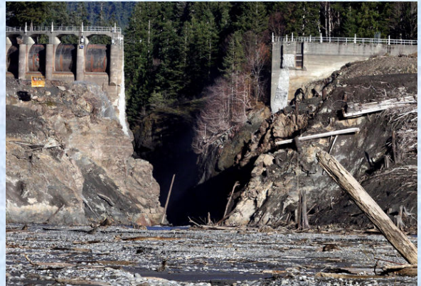
Glines Canyon Dam is two-thirds down, with the Elwha River pouring through the gap. Elwha Dam, 8.6 miles downstream, is already gone.
